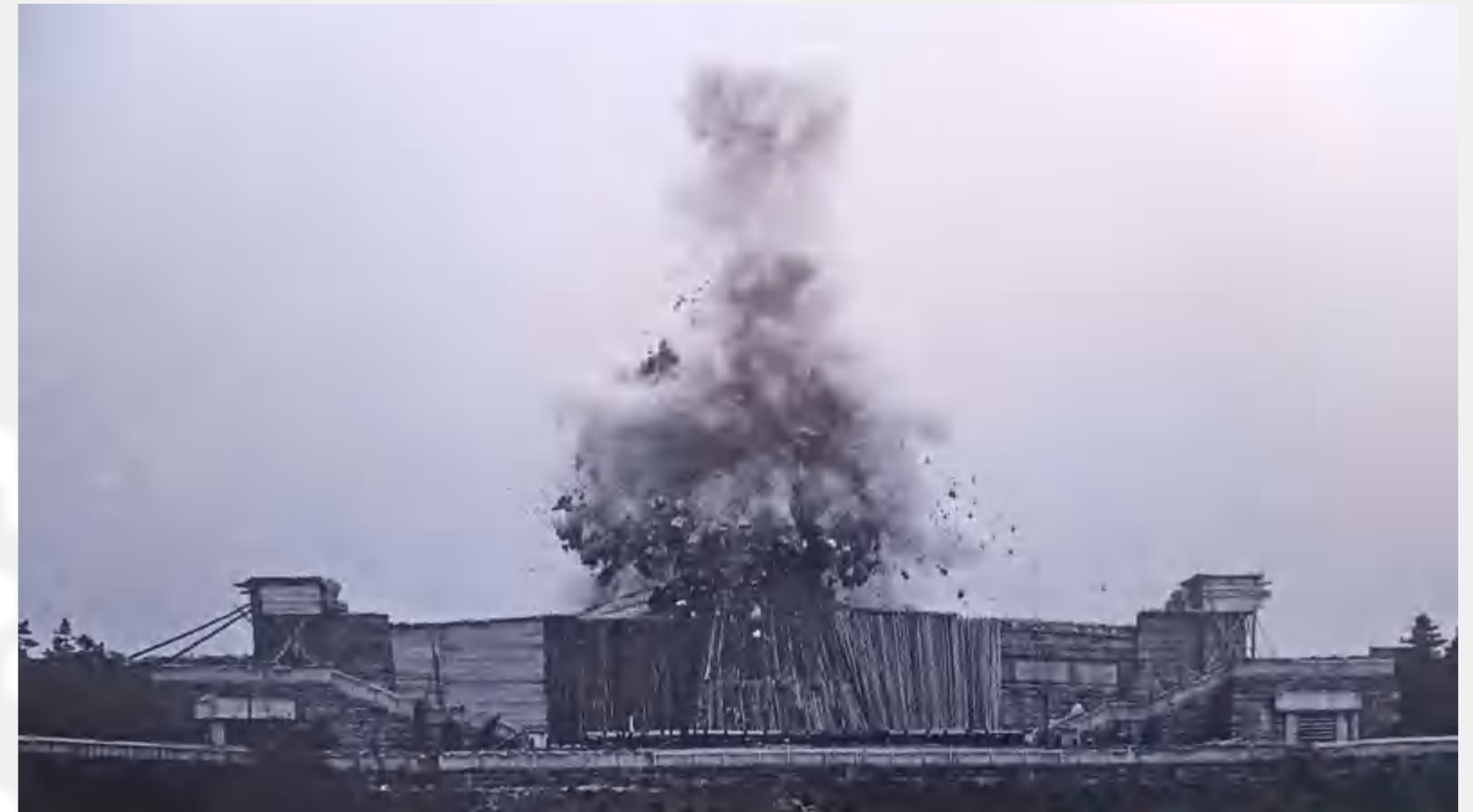
monument of Stalin that measured 15.5 meters high and 22 meters long with a bomb shelter created below it. It took 3 attempts to demolish it to the remnants of what it is today
