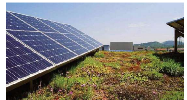
GREEN ROOF AND SOLAR PANELS
